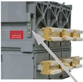
Figure 23a Circuit breaker identification block
